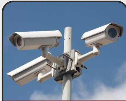
CCTV Surveillance System
