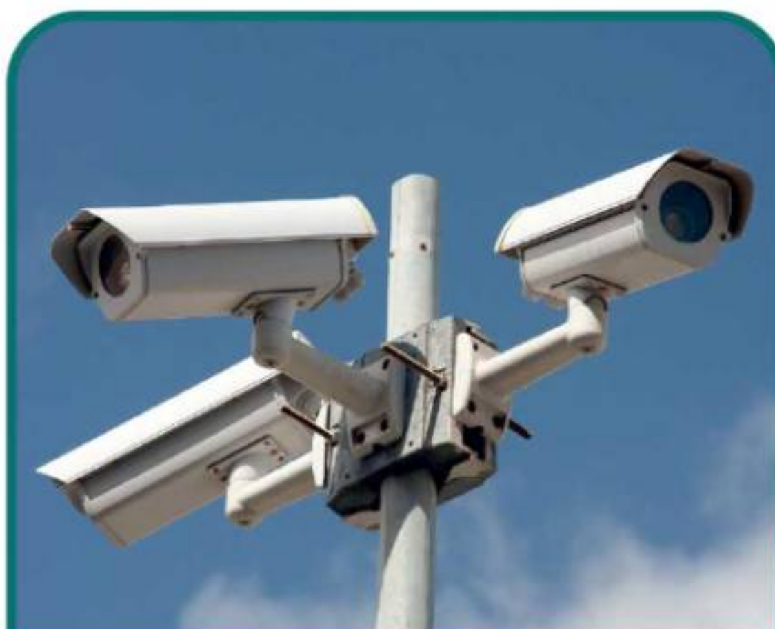
CCTV Surveillance System
