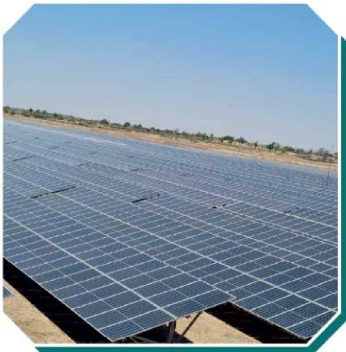
WORLD'S LARGEST SOLAR PARK (5000 MW)
