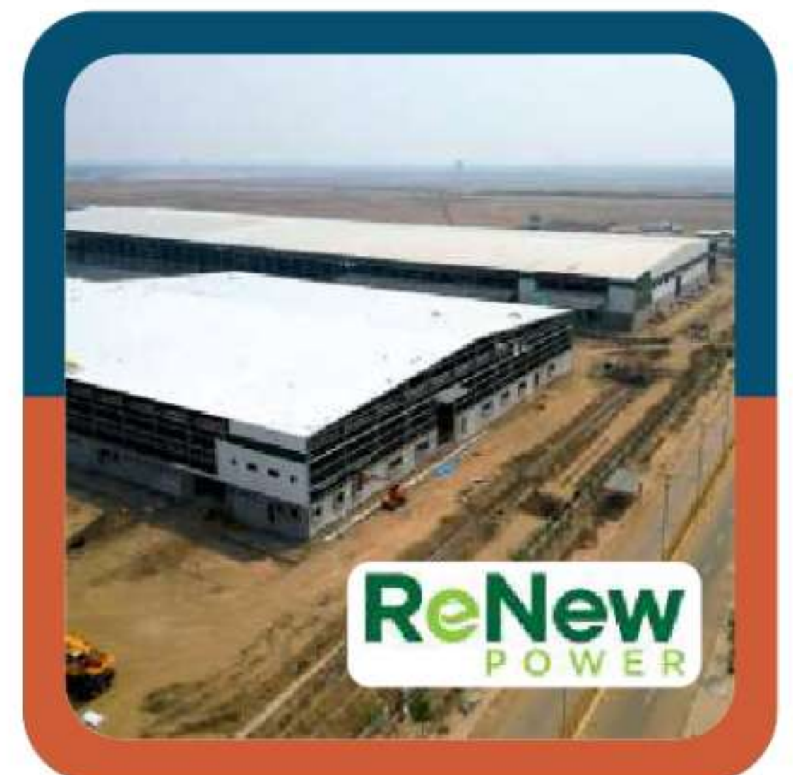
Renew Power - 2000mw Solar Cell 1200 Cr Construction Cost
